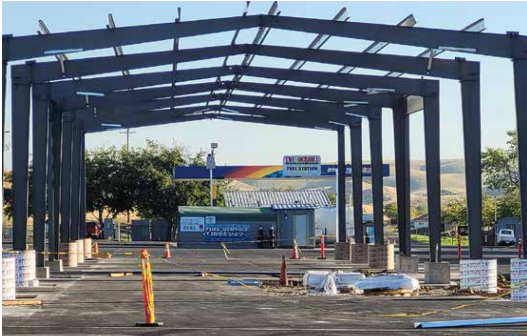
New Canopy in the paddock, notice the footprint left from the old store
