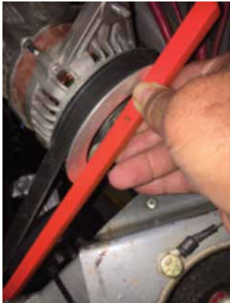
Alignment Bar at Alternator
